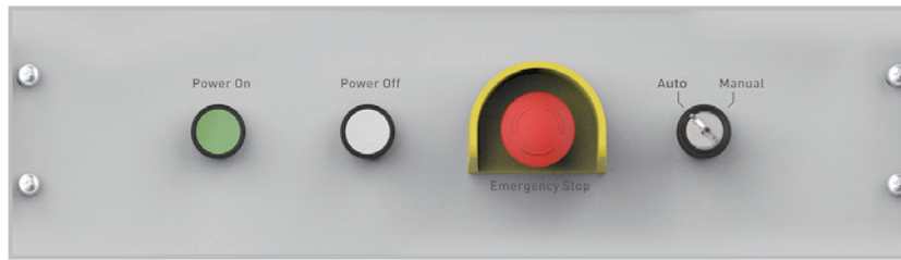
Rack Front Switch Panel (typical)
