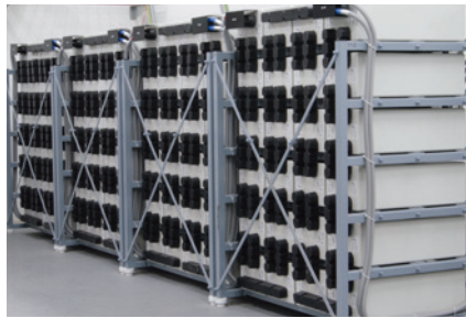
Energy Storage System
