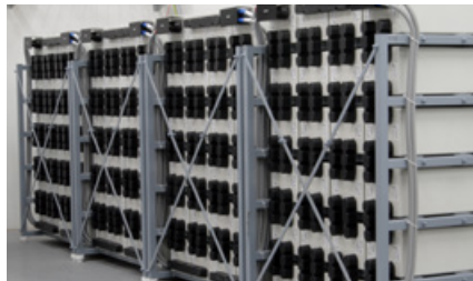
Energy Storage System
